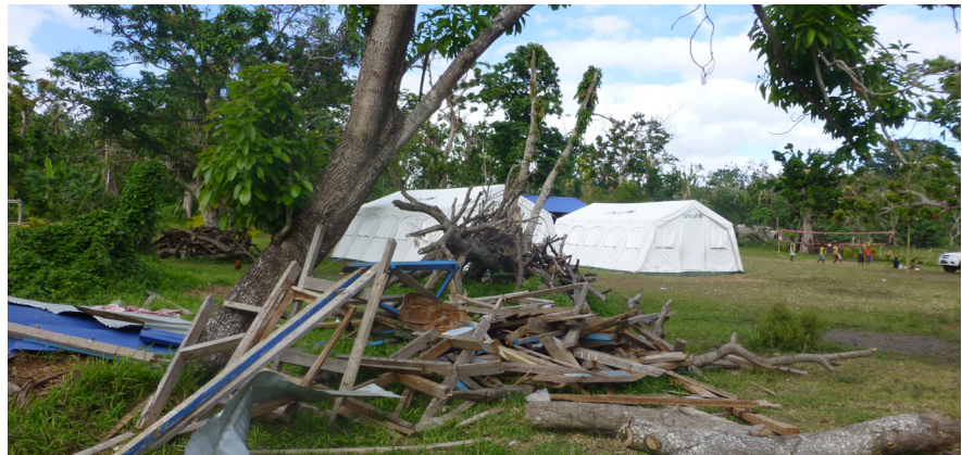
Damage and temporary classrooms after Cyclone Pam at Isla Mission School, Tanna. Isla has since been repaired and had classrooms rebuilt.
